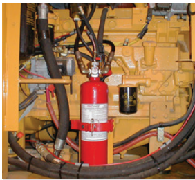
The red FIRETRACE cylinder can be seen here, along with the red detection tubing as it is run to the critical areas.
